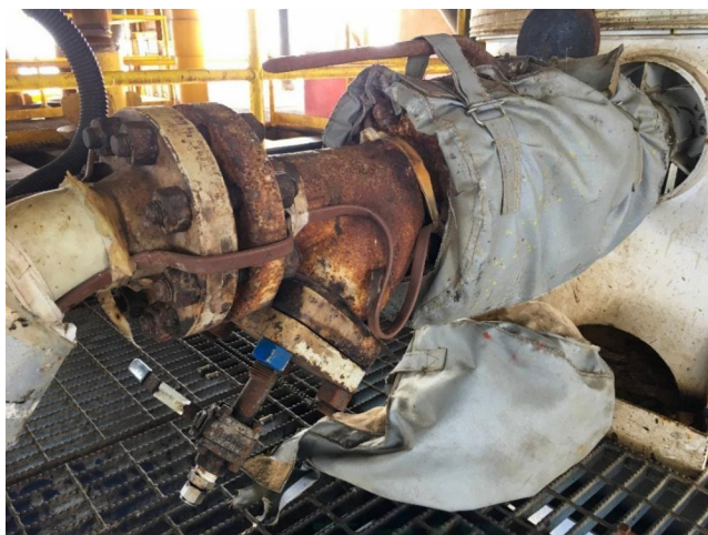
Fig. 2 Severe corrosion under insulation (CUI) in the piping system (Courtesy: Shutterstock)
