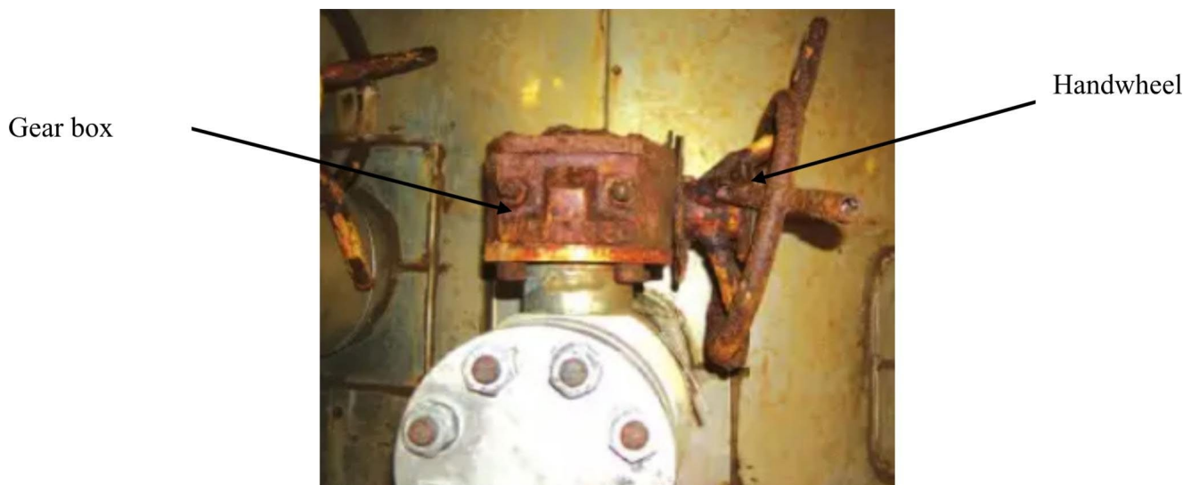
Fig. 5 Severe rust and corrosion on a valve handwheel and gear box made of carbon steel in the offshore environment (photograph by author)
