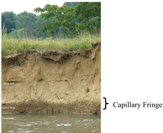
Fig. 3 The capillary fringe (dark discoloration above the water level) reflects the presence of high moisture content (more than 75% of the porosity). http://wps.prenhall.com/wps/media/objects/5309/5437119/Figures/chapter06.htm
