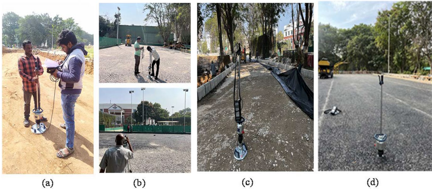
Fig. 4 Pictorial representation of LWD testing on a subgrade soil, b–c base layer (WMM), and d surface layer (DBM)
