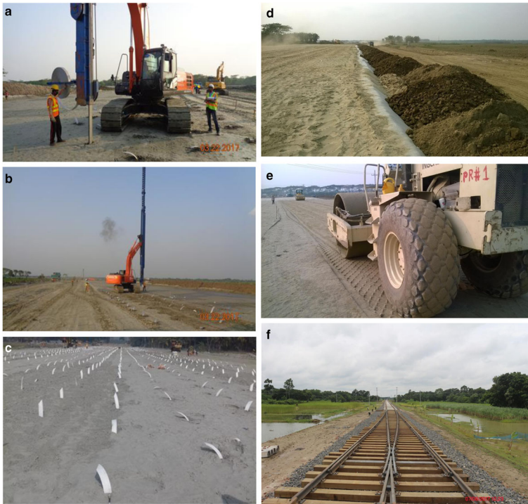
Fig. 9 a, b The installation of PVD. c The installed PVD. d First layer of sand blanket spread over the top. e Sand blanket is compacted with a vibratory roller. f The completed railway track
