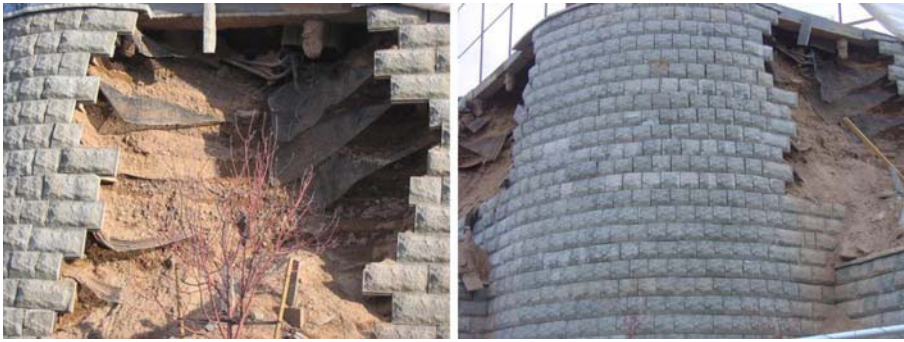
Fig. 1 Missing geogrids caused collapse one year after the end of construction: close up (left) and general view (right)
