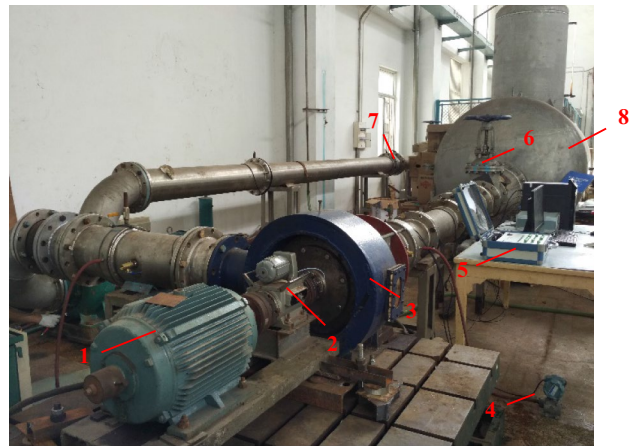
Fig. 9 Experimental device. 1) motor; 2) torque meter; 3) mixed-flow pump; 4) pressure transmitter; 5) HSJ2010 hydraulic machinery comprehensive data acquisition instrument; 6) inlet valve; 7) turbine flow meter; 8) water tank
