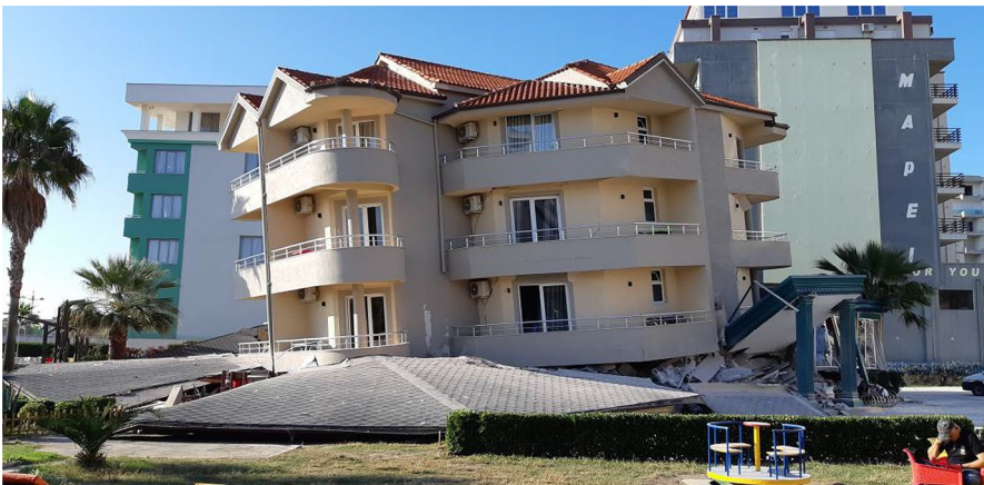
Fig. 18 Tilting of the building due to liquefaction and ground subsidence
