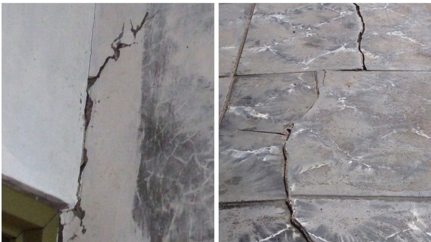
Fig. 14 The cracked wall and floor of houses located around 400 m from the measurement starting point
