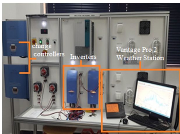
Fig. 5 Microgrid site in the laboratory
