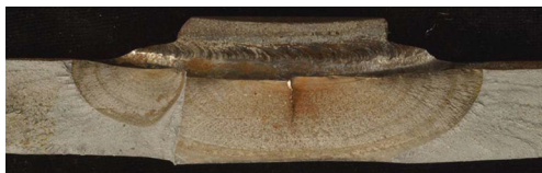
Fig. 15 Section through crack location 1 in specimen 3
