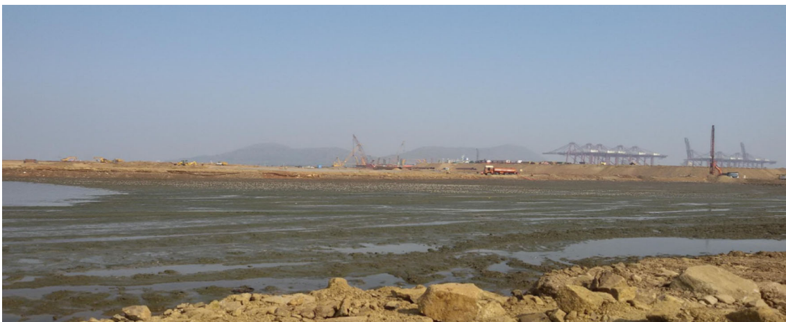
Fig. 12 Formation of mudwave ahead of the fill
