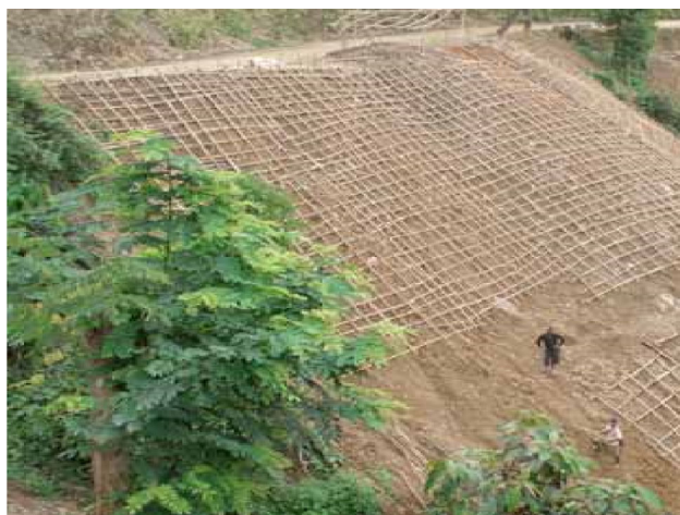
Fig. 18 Construction of bamboo knitting structures and plantation of local species of flora in progress [52]
