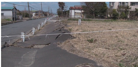
Fig. 1 A view of surface damage following floatation of a pipe line following the Tohoku earthquake of 2012 in Japan (Photo courtesy: Dr. SC Chian, National University of Singapore)
