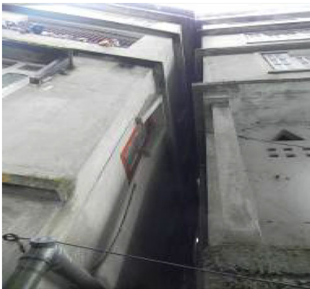
Fig. 10 Tilting of 2 adjacent buildings in “Seesa Gola, Gangtok”
