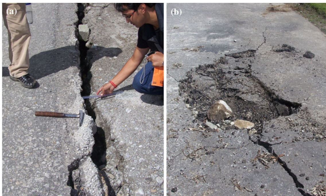
Fig. 8 Ground failure and damage to Roads in Lachung
