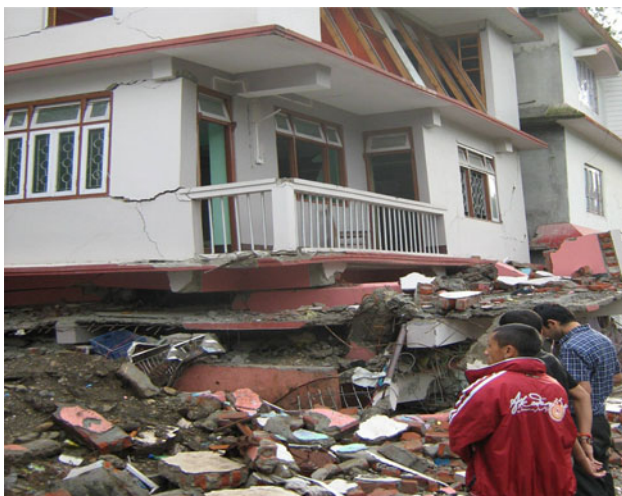
Fig. 12 Collapse of ground and first floor of a building in Jorhang (West Sikkim)
