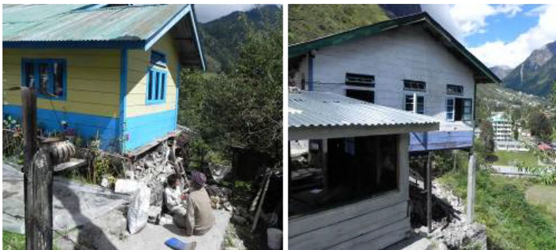
Fig. 13 Traditional light weight construction performed well except failure of foundation and supporting structure, Singring, Lachung (North Sikkim)
