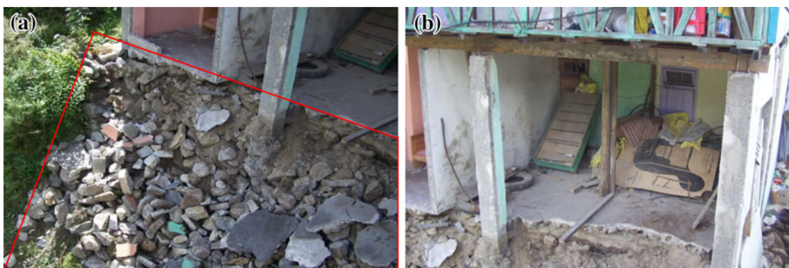
Fig. 6 Failure of a retaining wall (with red boundary) near Snowlion Mountain Resort, Lachung. (Color figure online)
