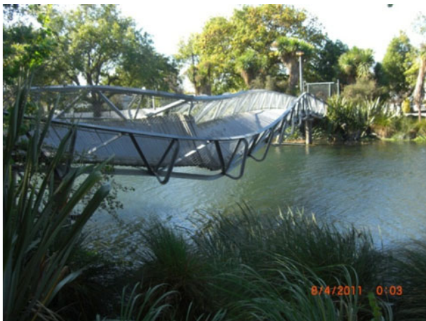
Fig. 2 Torsional buckling failure of a footbridge due to liquefaction-induced movement of the river banks
