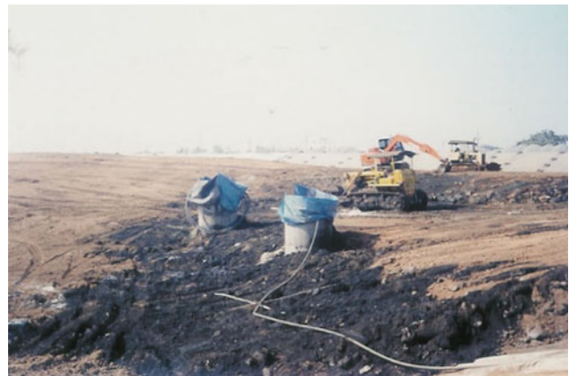
Fig. 11 Leachate collection wells
