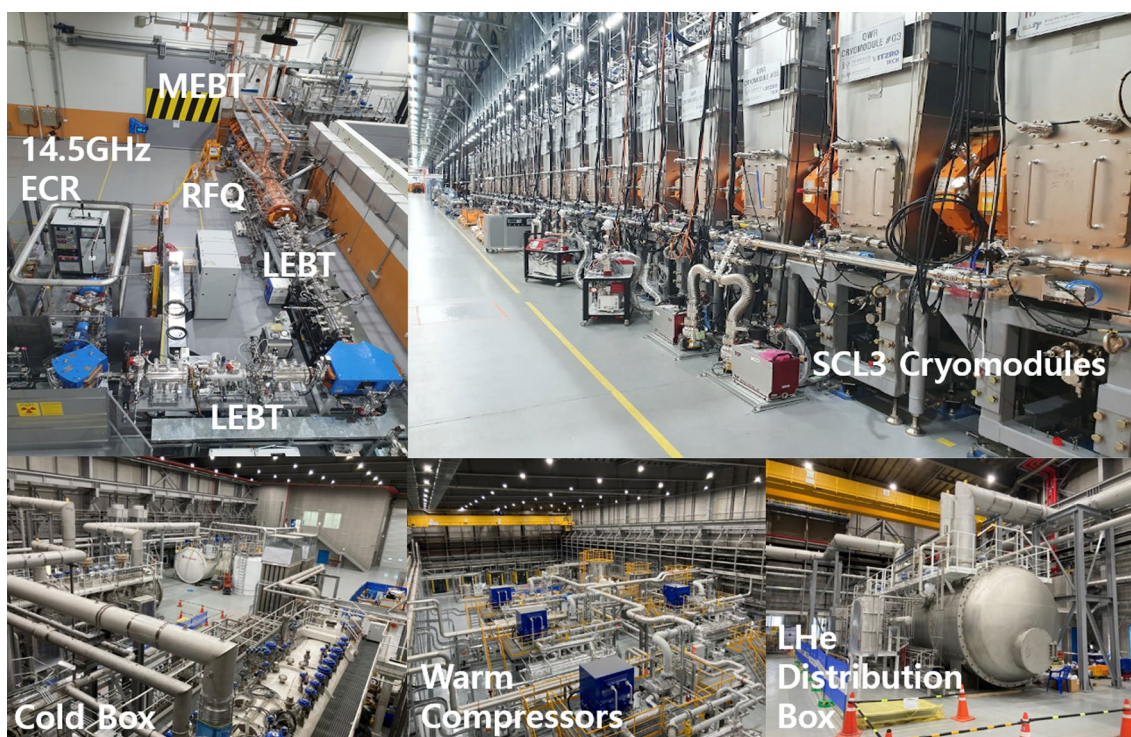
Fig. 3 Injector and SCL3 cryomodules in SCL3 tunnel and Cryoplants
