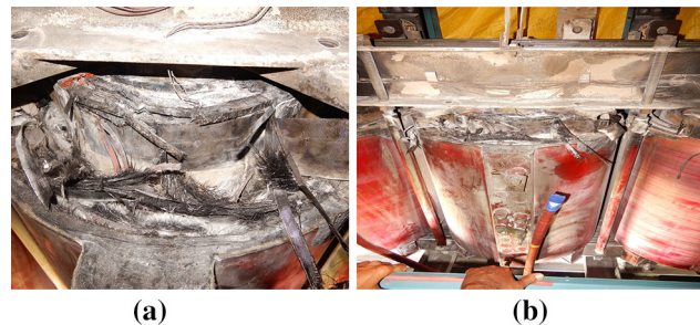
Fig. 2 a Failure of the insulation that came out from the transformer Y-phase winding. b Failed Y-phase winding insulation and winding top side view
