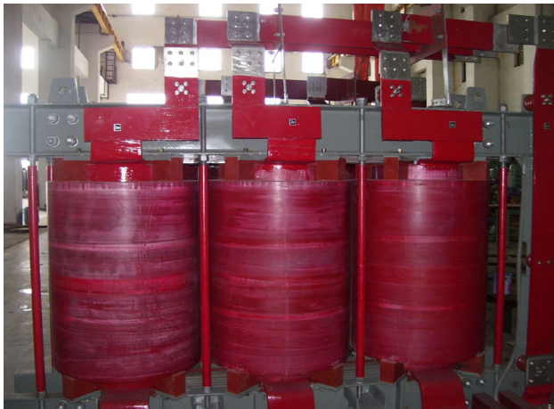
Fig. 1 Dry-type transformer assembly
