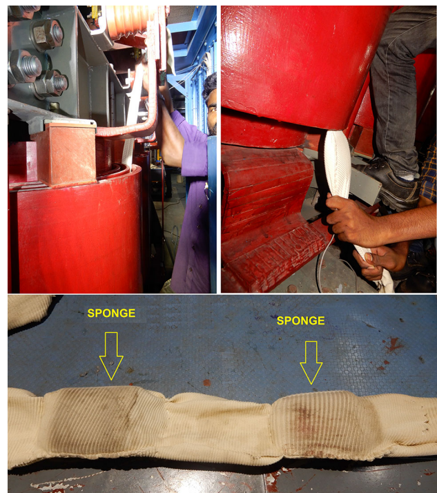
Fig. 4 Cleaning of the transformer winding using special cloth arrangement with sponge at higher temperature
