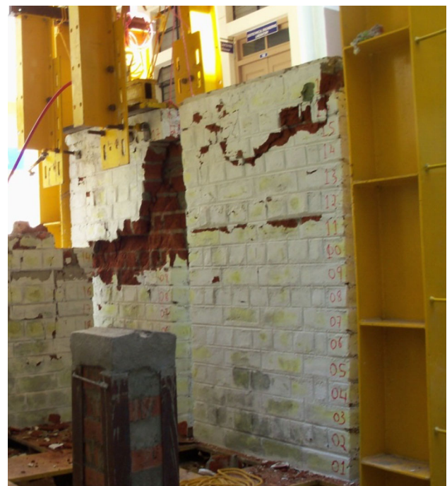
Fig. 6 Spalling in TMB-225-E-9 & TMB-225-E-10
