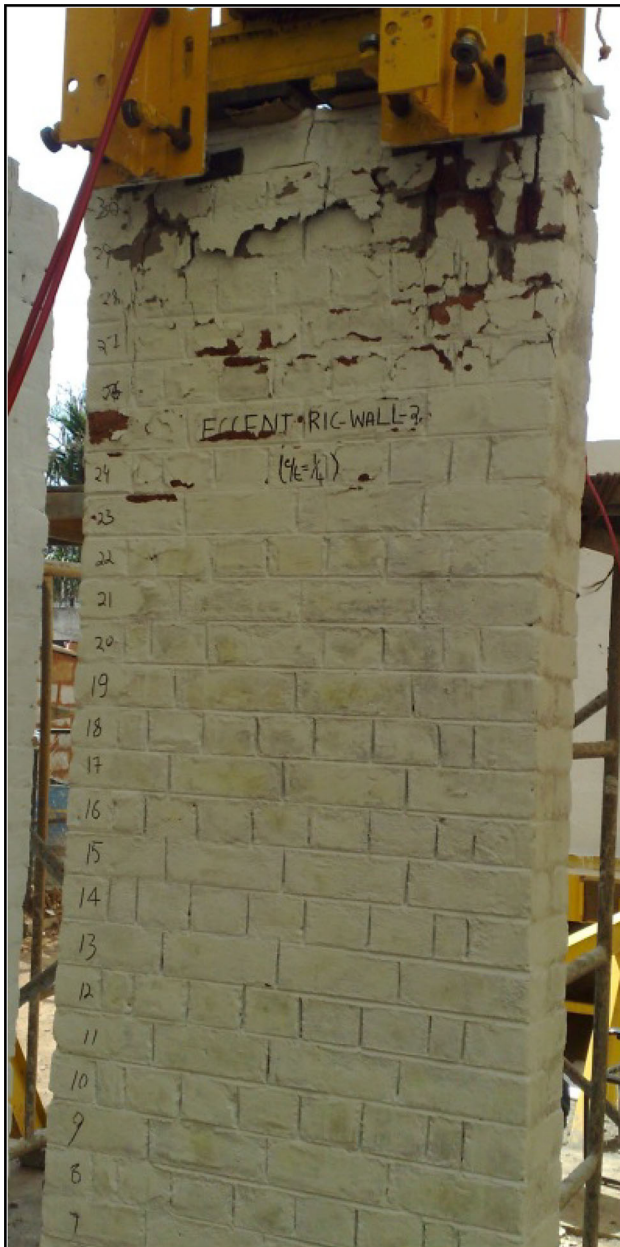
Fig. 10 Spalling in TMB-220-E-13
