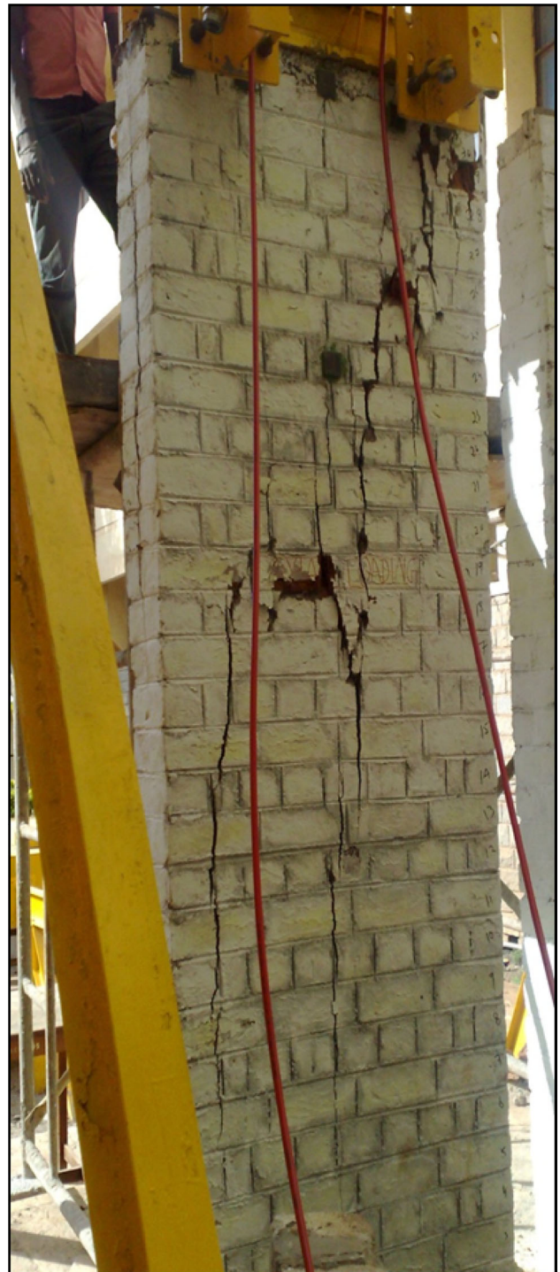
Fig. 9 Vertical cracks in TMB-220-A-4
