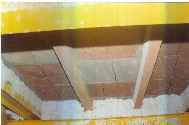
Fig. 8 Crack pattern in sand stone panels ( underside view )
