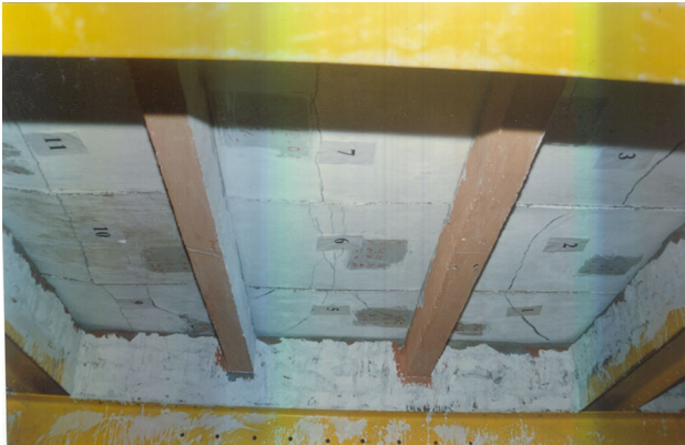
Fig. 7 Crack pattern in ferrocement panels with 20 % fly ash (underside view)
