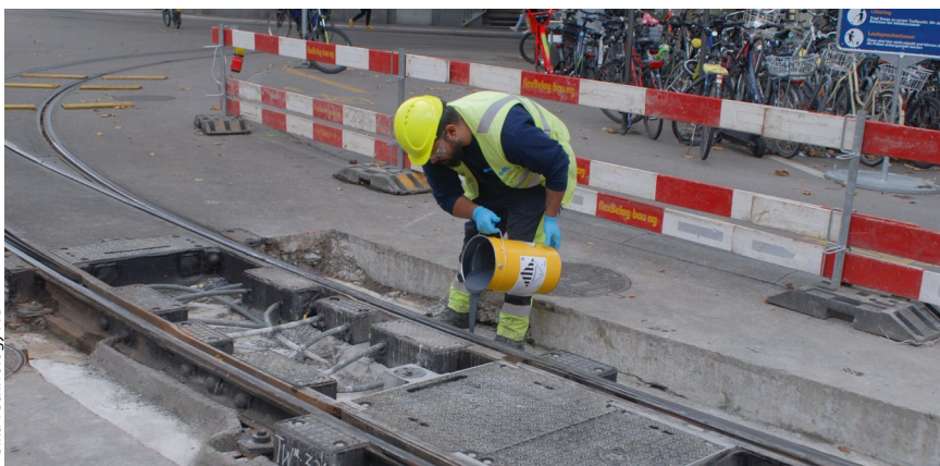
Figure 3 Mechanical (top) and manual application (bottom) of rail casting material on a transport infrastructure construction site.
