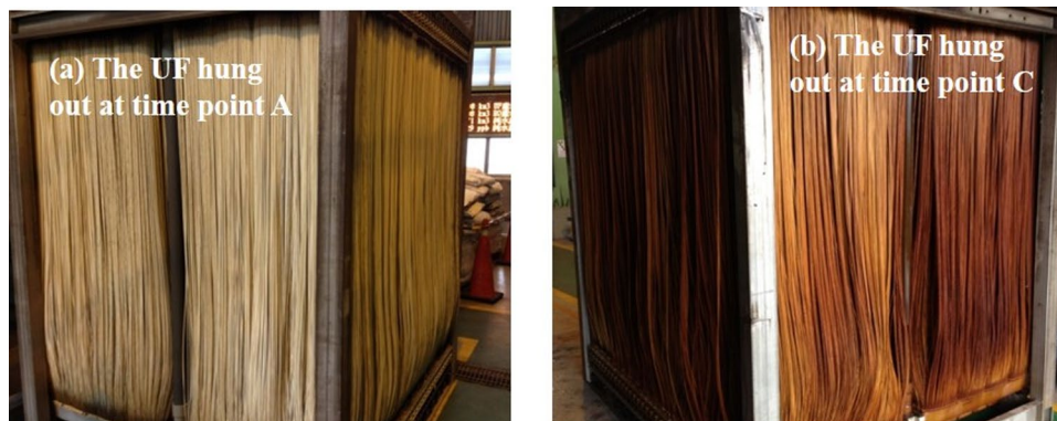
Fig. 3 Pictures of the same UF cassette in the IWPP hung out to clean and examine membrane fouling at time point A and C, respectively. The dimension of the cassette is 2561 mm (height) × 2136 mm (width) × 1744 mm (depth)
