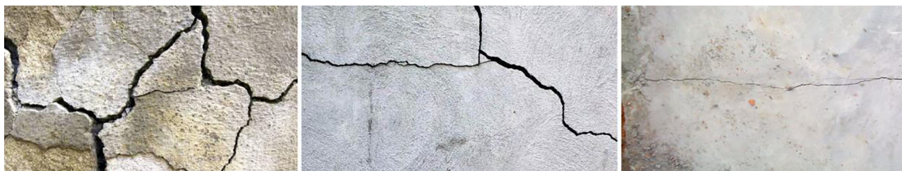
Fig. 2 Images of concrete surface cracks
