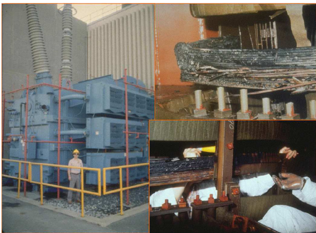
Fig. 4 Transformer damaged by an intense internal heating caused by the superintense 13–14 March 1989 geomagnetic storm. Left image : transformer under normal conditions. Two right images : details of the components whose melting down was caused due to severe GIC increases. Figure taken from Kappenman [23]
