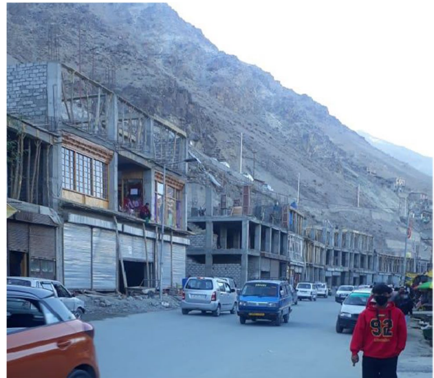
Fig. 7 Field photograph highlighting haphazard constructions coming along the base of a highly unstable slope (Kargil town)
