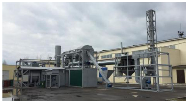
Fig. 1 Appearance of the FPP02 plant
