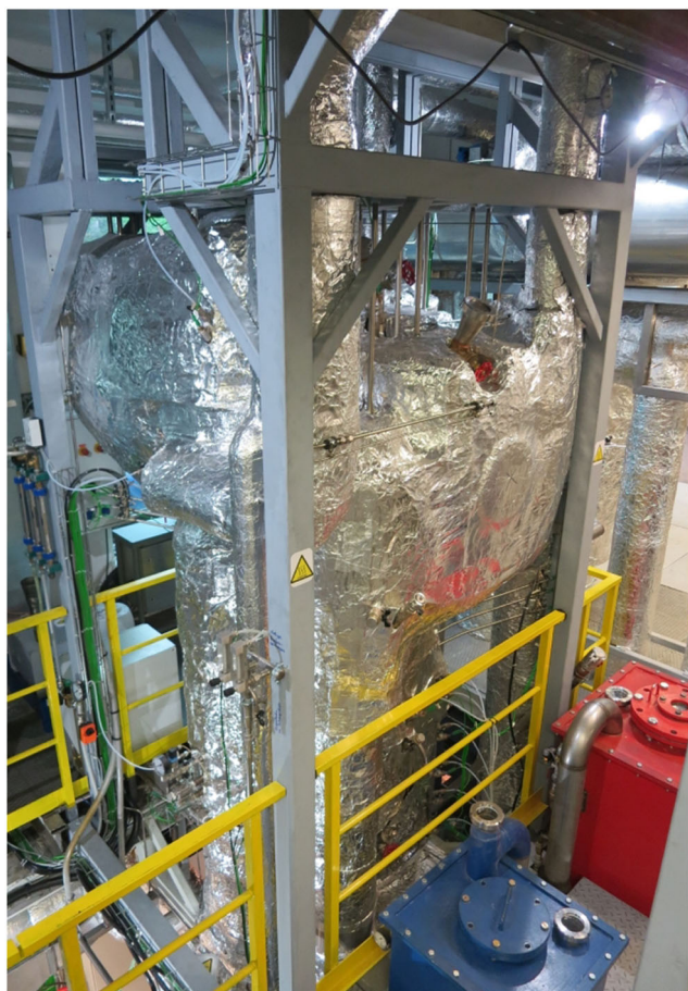
Fig. 3 Upper part of the 100 kW th gasification pilot plant, TU Wien [28]
