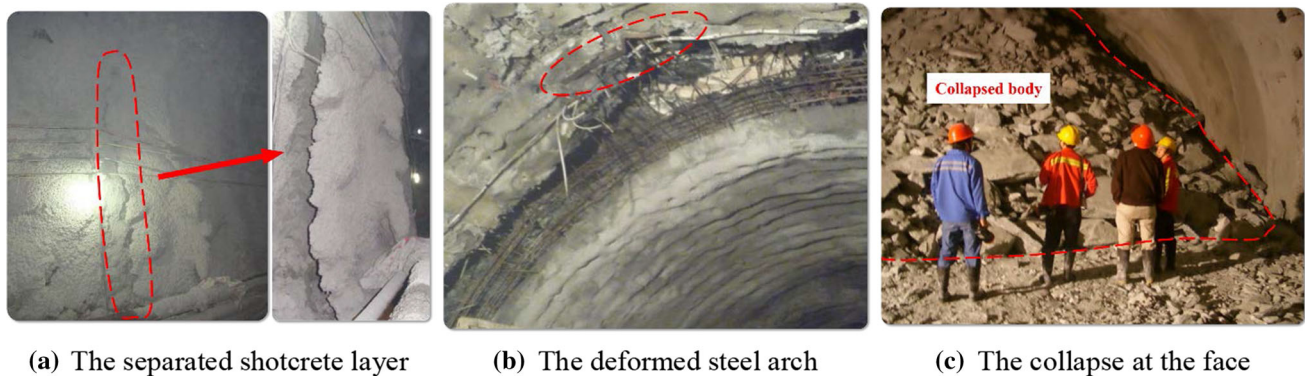
Fig. 28 Typical damage modes
