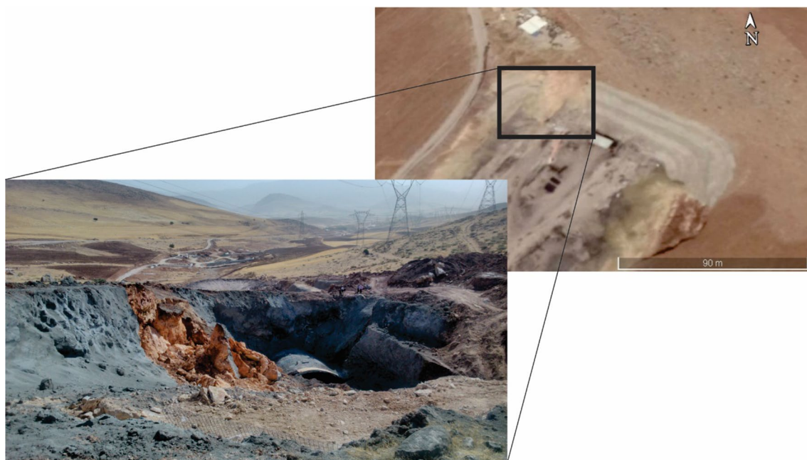
Fig. 4 Collapse at the outlet of the west tunnel (tunnel 1) due to the existence of weak rocks
