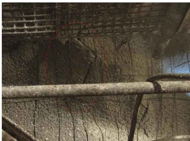
Fig. 10 Cracking occurs in potential risk zone obtained using MS monitoring
