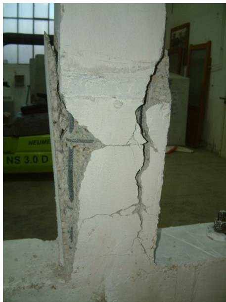
Fig. 11 Observed failure mechanism of the column C3C–BM–AF in experimental [16]
