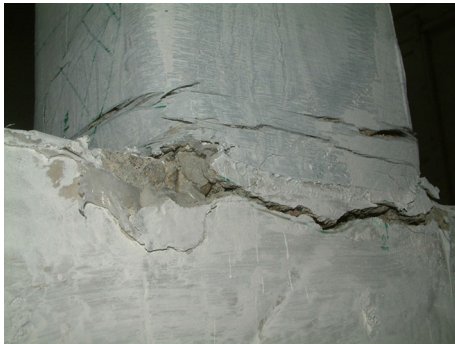
Fig. 14 Observed failure mechanism of the column C6C1–GW–AF in experimental [16]
