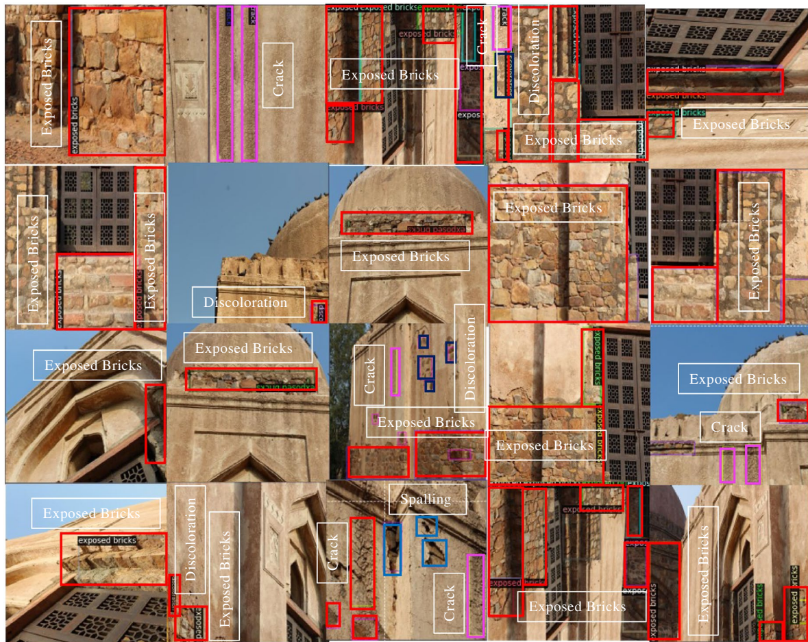
Fig. 2 Examples of data annotation. The data were annotated to identify four types of defects; spalling, crack, exposed brick, and discoloration
