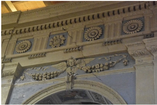
Deep crack on the South nave wall by the transept
