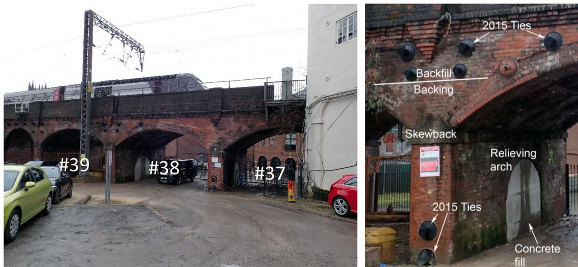
Fig. 1 Left—Northern view of the Marsh Lane Viaduct in Leeds, UK. Right—Closer view of the pier between Arches 38 and 39, showing the 2015 retrofit
