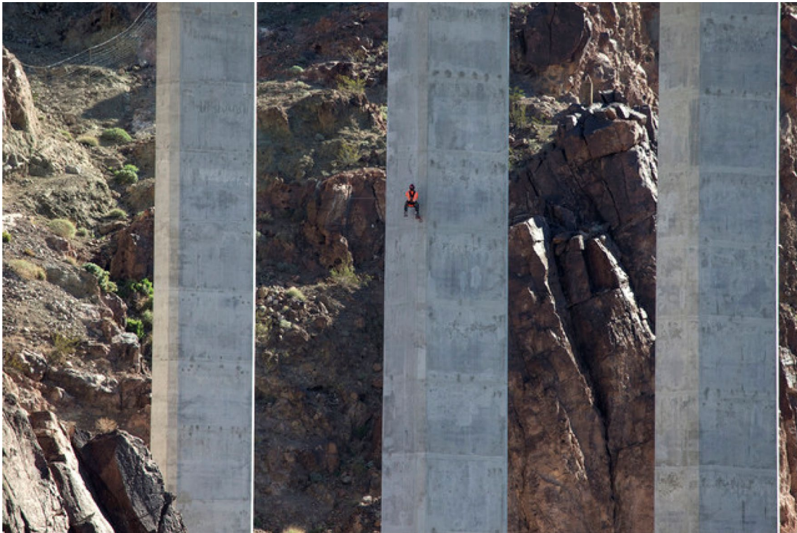
Fig. 1 Inspection of the Mike O' Callaghan–Pat Tillman bridge for deficiencies at the Hoover dam
