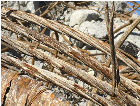
Fig. 6 Polcevera Viaduct: pitting corrosion of prestressing tendons [3]
