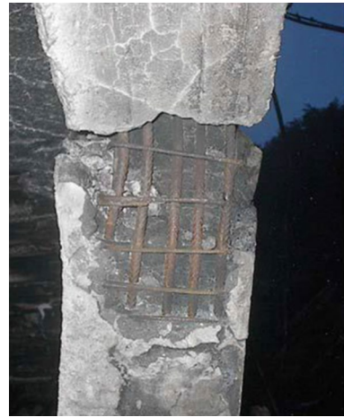
Fig. 15 Damage on RC structural elements caused by the earthquake of Santa Venerina in 2002 [12]
