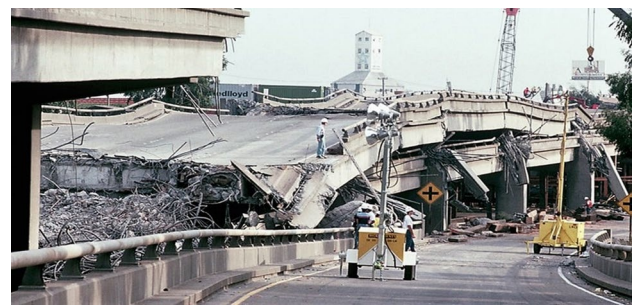
Fig. 8 Cypress Street Viaduct collapse [5]
