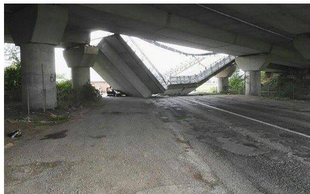
Fig. 4 The viaduct collapsed at Fossano, Italy
