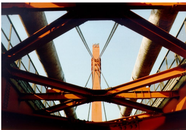
Fig. 3 Cables fanning from one of the steel pylons (view from the walkway)
