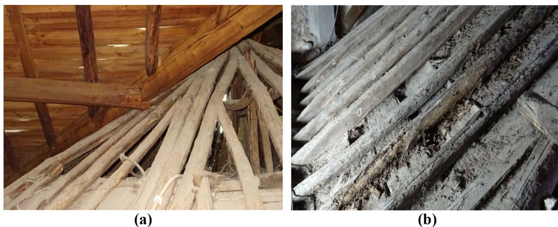
Fig. 9 Beam of the northern roof structure pressing the top of the octagonal dome (a). Severe insect wood deterioration on the external surfaces of the joists from panel V (b)
