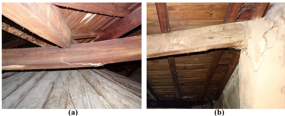
Fig. 13 Tensile crack of the horizontal beam (11) under excessive bending (a). Collapse of the purlin (42) due to the failure of the masonry support (b)
