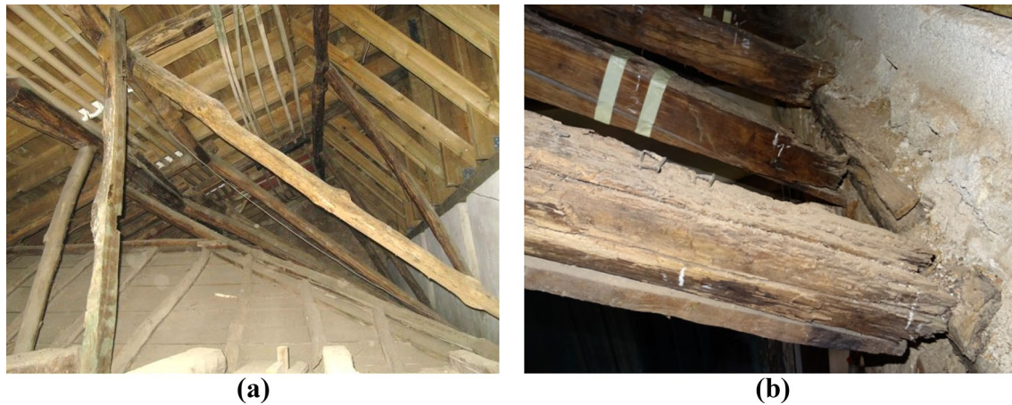
Fig. 6 Coexistence of old and new timber roof structures above the dormitory Room 68 (a). Rafters featuring insect wood deteriorations on their external surfaces and fungal decay at their ends (birdsmouth joint) with the wall plates (b)
