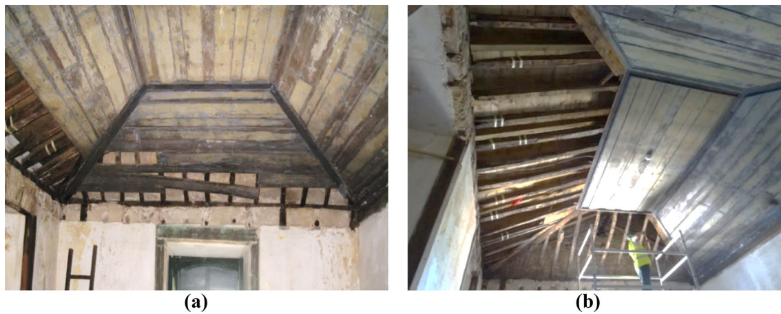
Fig. 4 Western rafters and northern joists made visible before (a) and after (b) removing the ceiling planks
