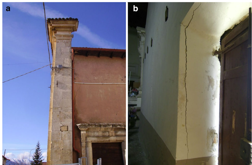
Fig. 5 Incipient overturning of the main façade (a) and horizontal bending mechanism of one of the longitudinal walls (b) of the church
