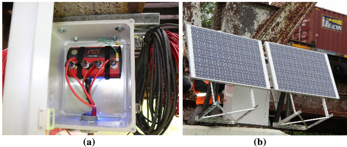
Fig. 3 Deployed monitoring system: a BDI node; b solar panels
