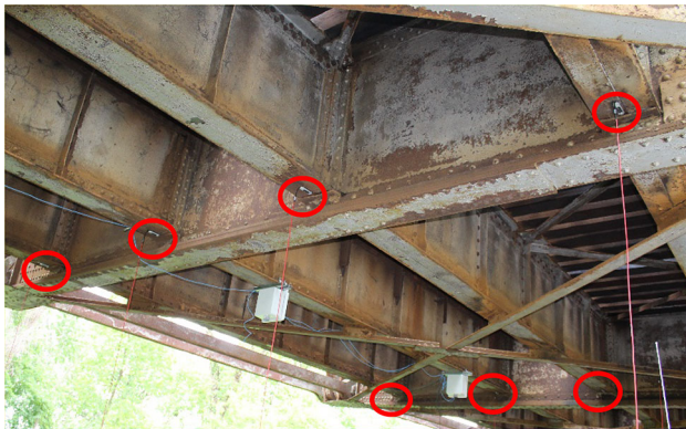
Fig. 4 Installed strain sensors (circled)
