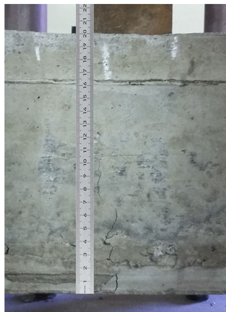
Fig. 13 Crack of Beam 02
