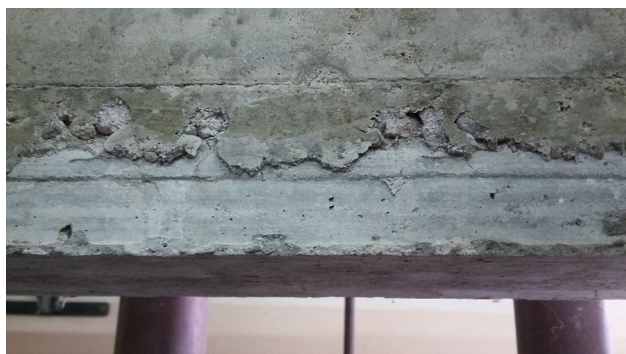
Fig. 12 Zone of the crack in Beam 01 after unloading. The crack is closed and not visible
