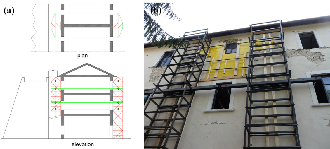
Fig. 4 Provisional interventions carried out on SE and SW wings: connection of the internal and external façades by means of steel cables and frames
