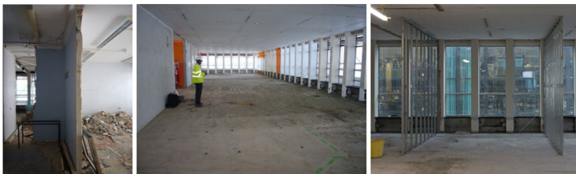
Fig. 3 Half-demolished masonry partitions, cleared floor and lightweight steel frames for new fixed partitions
