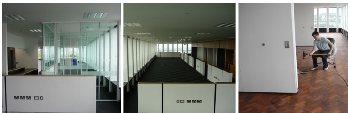
Fig. 4 Post-retrofit partition arrangements. Level 7 ( left ) full-height glass and half-height cantilever, level 8 ( middle ) half-height only and level 18 ( right ) movable partitions retracted, with hammer test in progress
