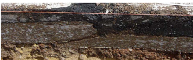
Fig. 3 Example of “stepping” in a road pavement caused by mining induced compressive strain.
