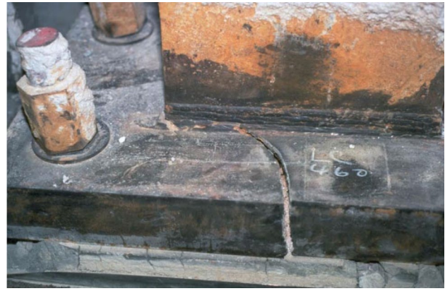
Fig. 1 Fracture of 100 mm thick base plate created by overturning moments in braced bays following 1994 Northridge earthquake: These fractures appeared to start at the fillet welds connecting the columns to the base plates (Bertero et al. 1994)
