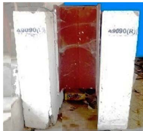
Figure 7. Concrete crushing and separation of slab.
