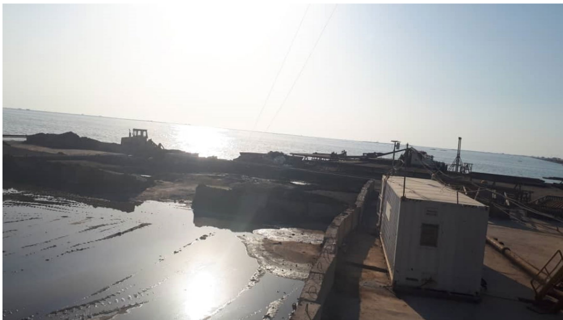
Fig. 5 Reed vegetation is gone in the drilling field next to the Hawizeh Marshes
