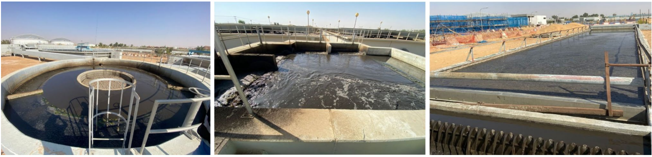
Fig. 1 Waste Water Tertiary Treatment Plant at Hail. The TSE could be stored to be utilized further in case of emergency
