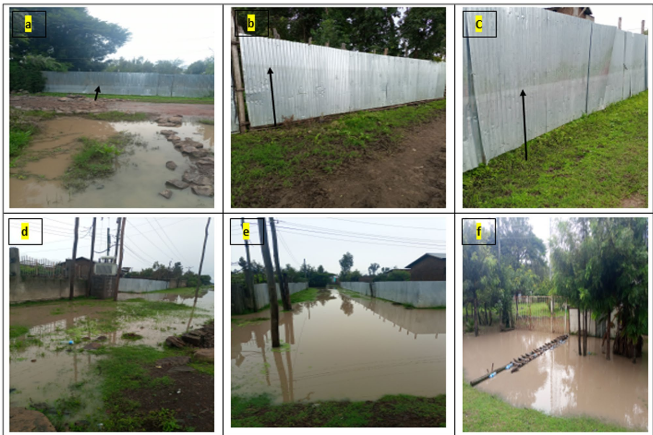
Figure 13 Flood marks of 2019 river flood event in (a), (c) in Teji and (b) in Asgori towns, and (d, e, f) flash flood on Teji town around Ilu Police station and Hidasie Telecom 2021
