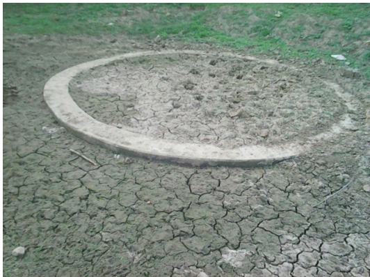
Fig. 13 Clogged RW along with silted Canal bed at Godagari
